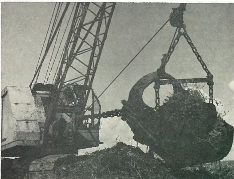
ONE OF THE LEAST glamorous, yet most important methods of conquering mosquitoes is through dragline operations, which cut new drainage canals and impound water via dike buildups.
