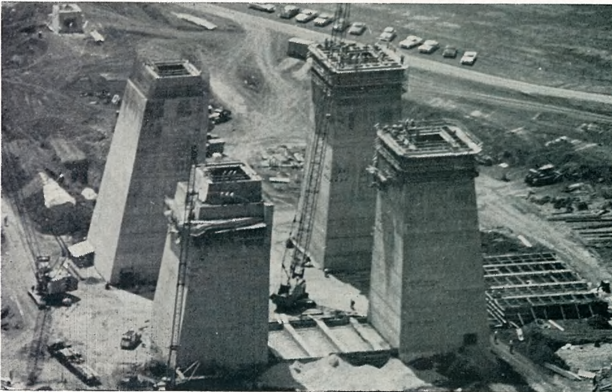
FOUR GIANT CONCRETE pillars, vaguely resembling an Egyptian pyramid, form the lower sections of a Saturn booster static test stand at MSFC. The legs will reach 144 feet in height and will be topped by a steel superstructure and boom crane. The $30 million complex, which at its construction completion next year will stand 405 feet high, will be first used for a captive test in August 1964.
