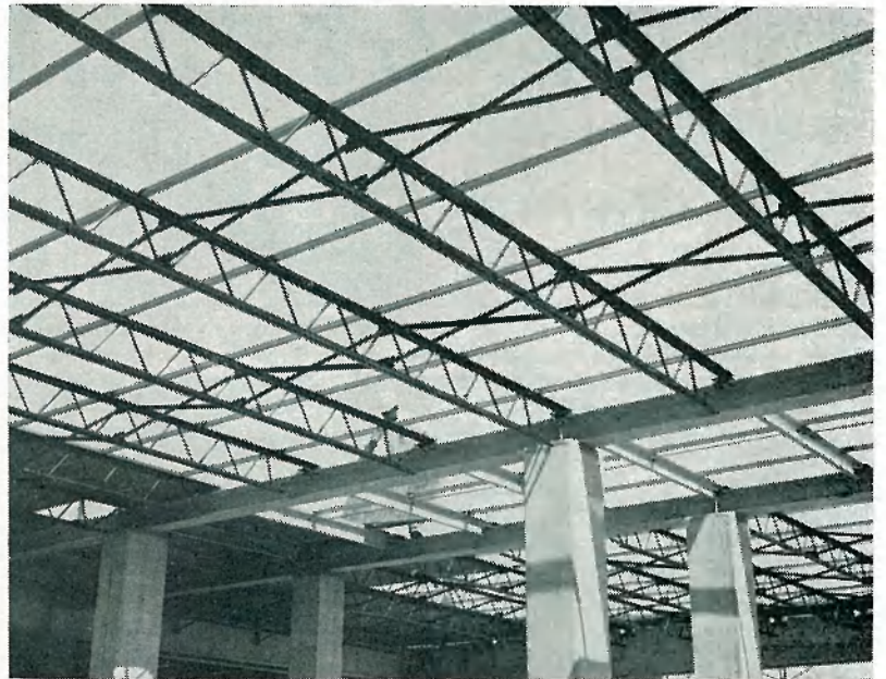
LATTICE-WORK of steel beams changes daily as construction work on the addition to the E and L building nears completion. Scheduled for occupancy early next month, the new wing will provide 13,760 square feet of space for engineering offices.
