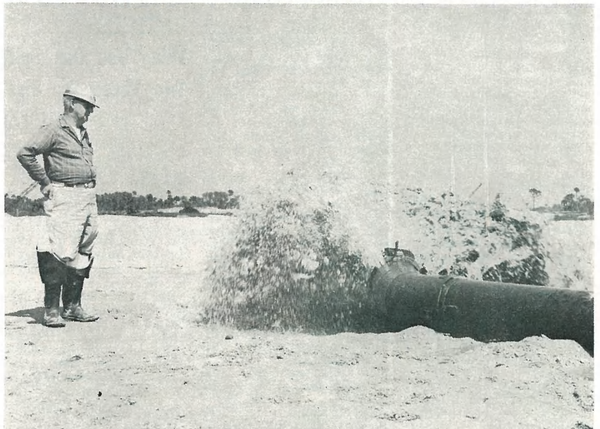
AFTER BONES were found from a now extinct species of elephant, the U. S. Corps of Engineers requested the Gahagan Dredging Company to post a workman at the end of the pipe from the dredge Overland — to spot any additional fossils that might be pumped out.
