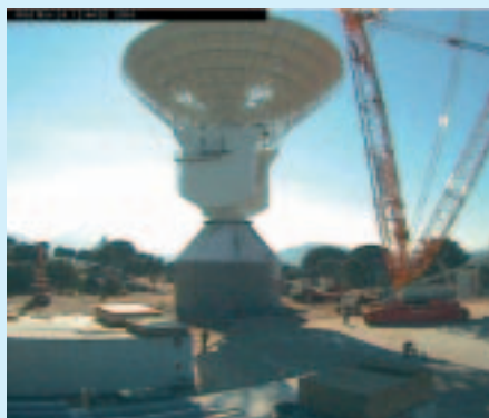
Mounting of the antenna dish at ESA's Cebros deep-space ground station in Spain
