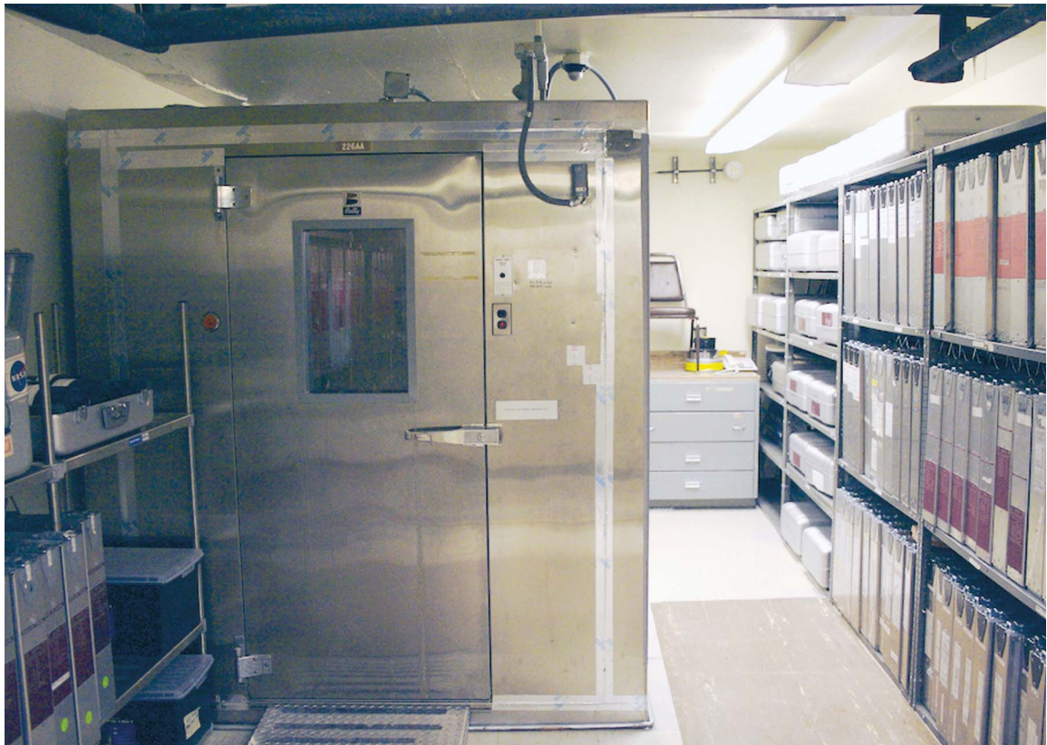
THE FREEZER IN BUILDING 8, JSC, HOUSTON
