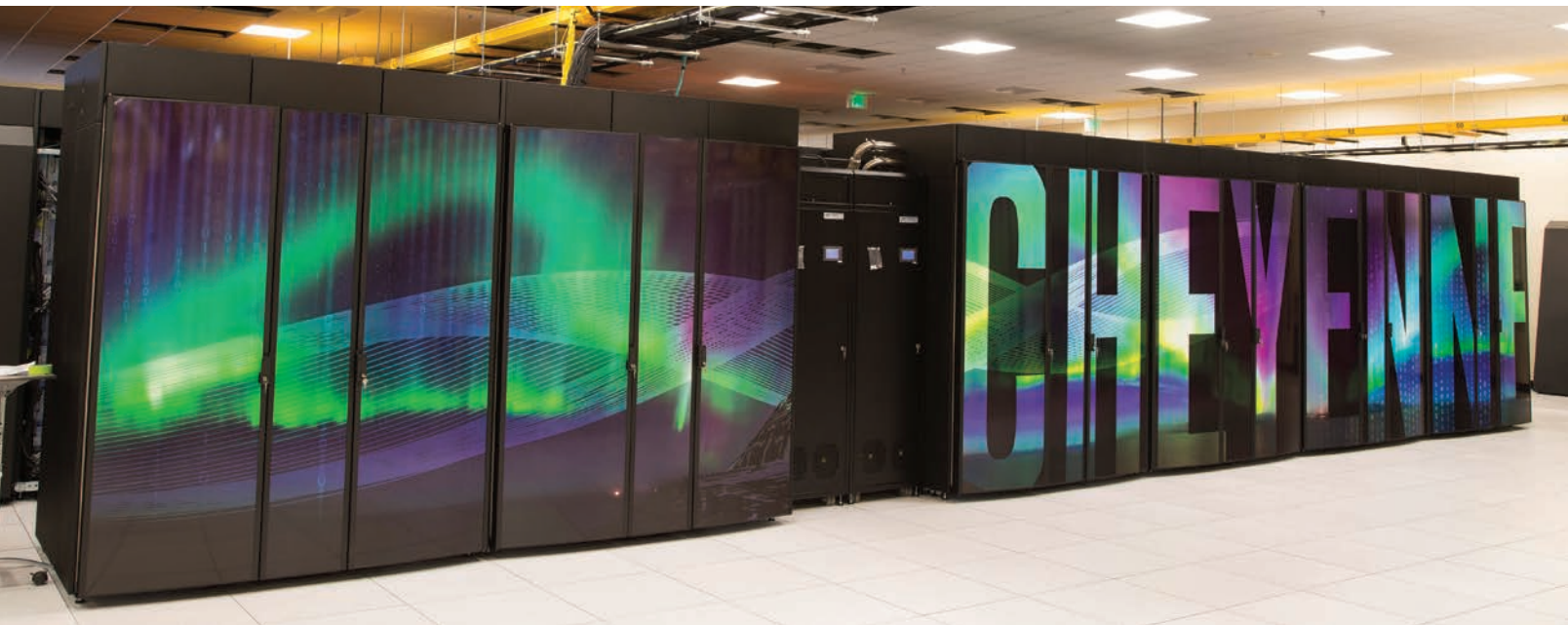
The central processing unit-based Cheyenne supercomputer, went into service in 2017 at the National Center for Atmospheric Research (NCAR)-Wyoming Supercomputing Center. Credit: University Corporation for Atmospheric Research (UCAR), Carlye Calvin, CC BY-NC 4.0 ( bit.ly/ccbync4-0 )
