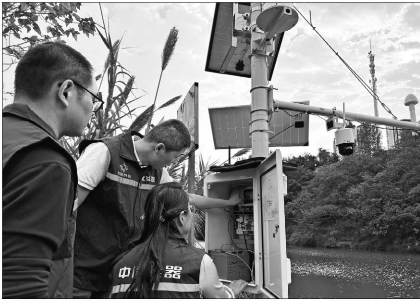
Technicians from BeiDou Satellite Communication Co Ltd conduct on-site equipment debugging at the Longjiansi Hydrological Monitoring Station in Luzhou, Sichuan province, in July. PROVIDED TO CHINA DAILY
