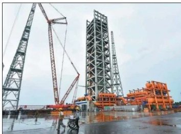
Workers put the final touches on the second launch service tower at the Hainan International Commercial Aerospace Launch Center in Wenchang, Hainan province, on Thursday.
