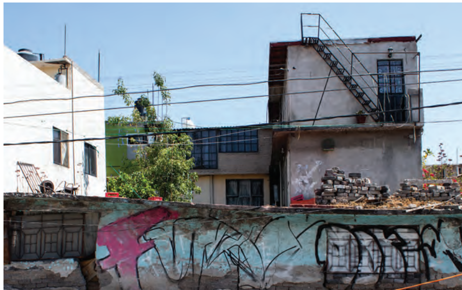
In the Ampliación Santa Martha neighborhood of Mexico City, land subsidence has contributed to hundreds of leaning fences, fractured walls, and cracked streets. Credit: Rodrigo Botello
